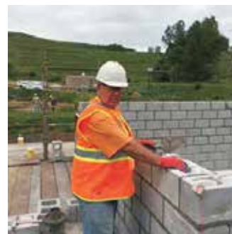
Kurt Deitman @ Homer City Power Plant
